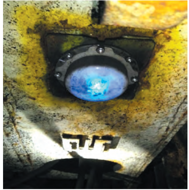
Fig. 8. Sensor installation in real-life conditions using mounting brackets
