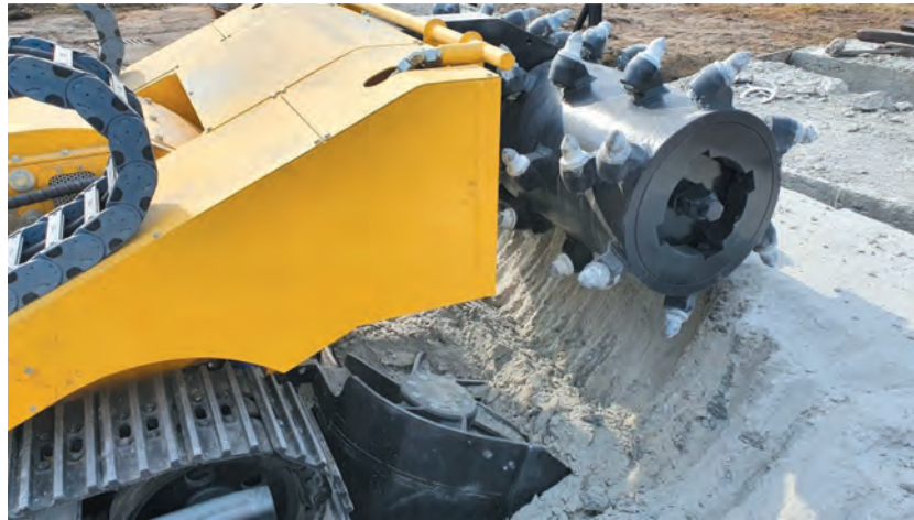
Fig. 3. Operation of floor grinding machine – grinding of blocks with chunks of floor rock on the testing ground
